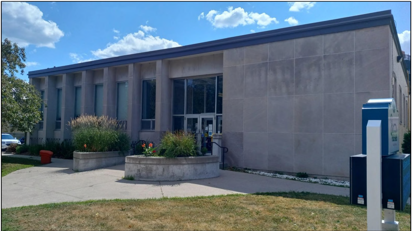
Completed in 1967 as a Centennial project, the former Oxford County Library Headquarters building still stands at 93 Graham Street in Woodstock. It housed library administration plus a small circulating collection until 1997. Drill holes and other scars on the building's front reveal the sign that once was: "Oxford County Library". Today, this building houses Southwest Public Health. Photo taken in July 2022.
